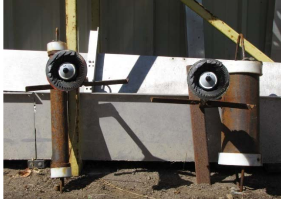
Figure 2.9. A 4-in.-diameter trolley with hydrophone (left) for slotted pipes on powerhouse piers and an 8-in.-diameter trolley with hydrophone (right) for slotted pipes on spillway piers. Each trolley had a steel arm to support a hydrophone that was surrounded by a plastic cone lined with anechoic material to prevent sound reception from a downstream direction.
