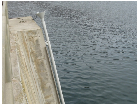
Figure 2.8. Trolley pipe mounted on a main pier of the John Day Dam powerhouse
